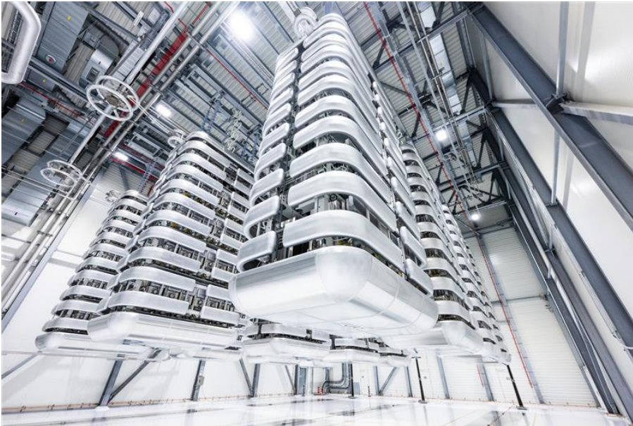
Plate 5-14 Indicative Image of the Inside of a Valve Hall
